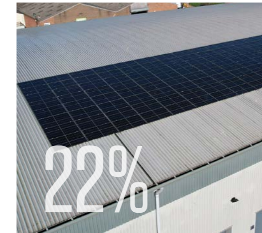
UK office energy generated by solar panels.
